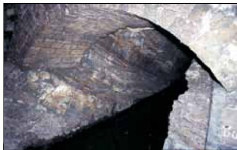
Peering into the Canal Tunnel from a cross-heading bridge; brick arching supports the largely natural rock section.
