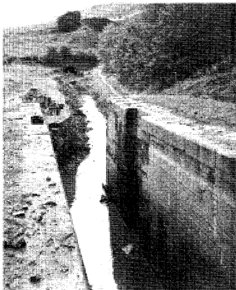
Lock 12W to Scout Tunnel. The lock chamber has been emptied and the channel cleared to reveal the washwalls.
