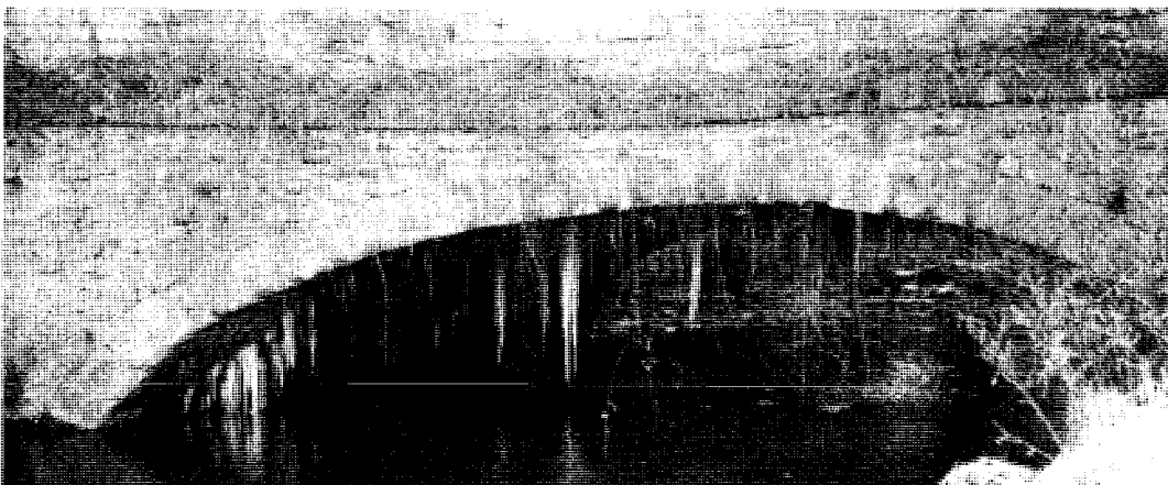
"Owd Sag" aqueduct, Dobcross. Scheme No. 8 in the work list. If anyone is still in any doubt that Owd Sag is leaking.....!
