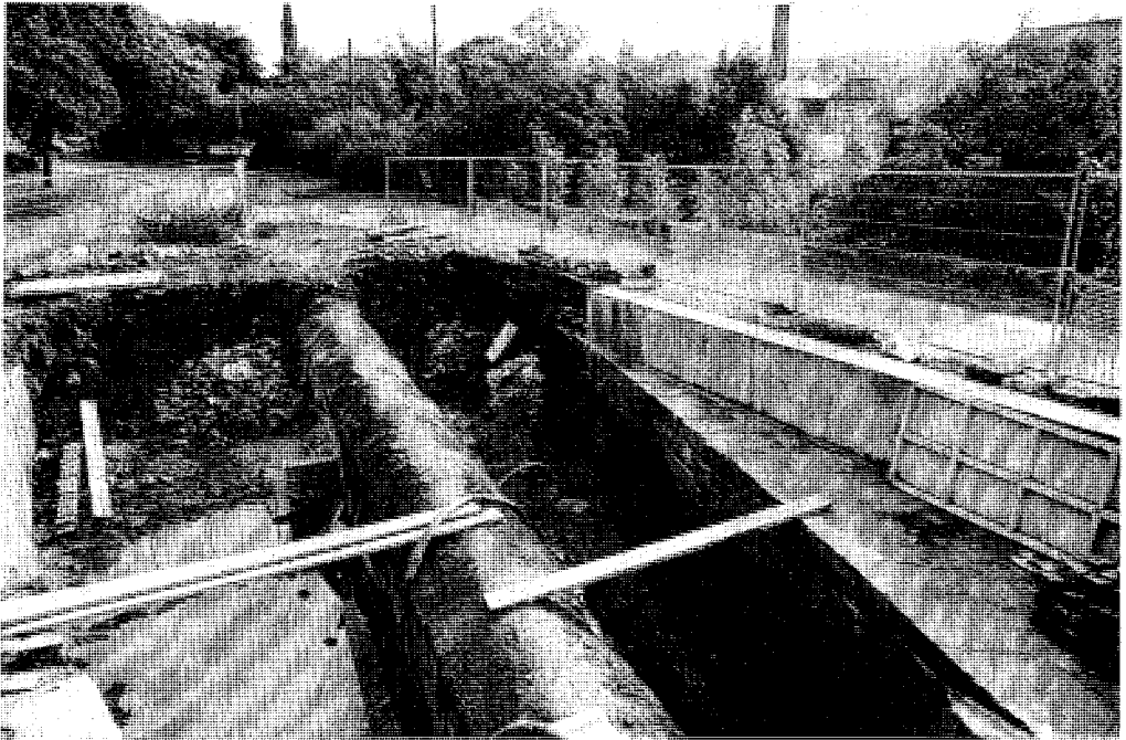
The new concrete retaining wall to the road to the Manor House and car park below Lock 23E, Slaithwaite.
