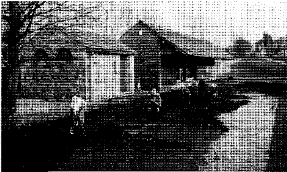
Above: Waterways Recovery Group (WRG) get stuck in at the Wool Road Transhipment Warehouse, or maybe they're planting themselves to grow more volunteers? Photo: K. Wright
