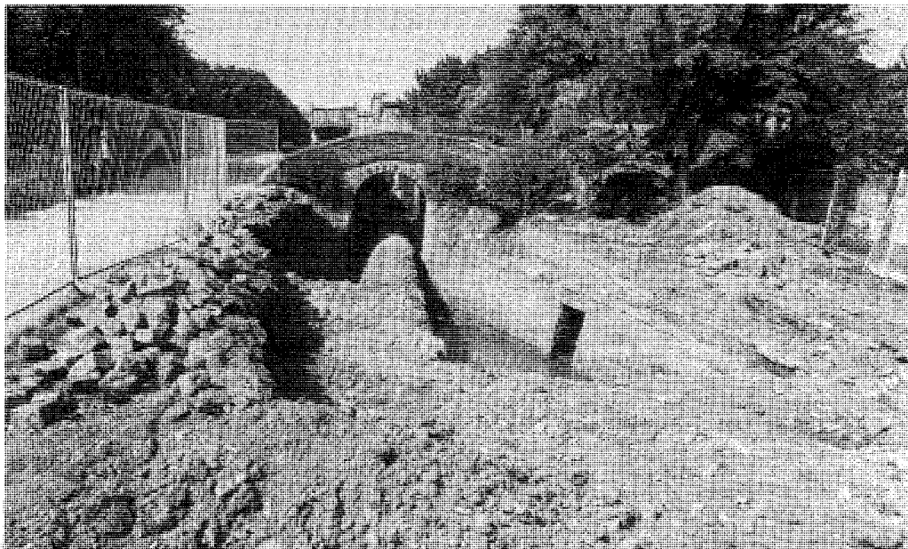
Lock 23E, Slaithwaite. The lock chamber, beyond the footbridge, is being dug out, whilst preliminary excavations have revealed the bywash exit in the washwall. The central culvert pipes the canal through the town centre infill. It is planned to create a small pound this side of the lock allowing a section of obstructing culvert to be removed. Photo: R. Gough
