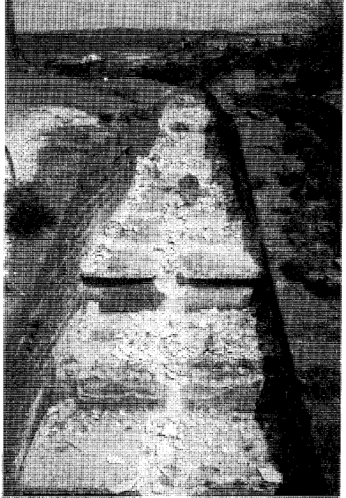
Lock 29W, Diggle. The concrete capped cascade is ready for excavation. Photo: A. Ogborn
