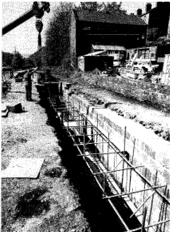
Lock 24E, Slaithwaite - The offside chamber wall is almost rebuilt bar another course and the copings. Restoration staff John Francis (guiding bucket) and Barry McDonald (down below) set to on the nearside wall. Photo: R.Gough
