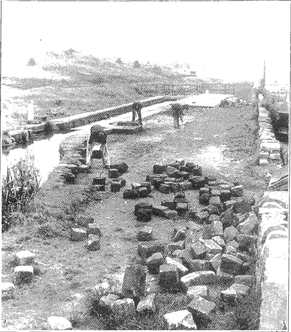
Original landscaping work taking place in 1974 after the chamber had been infilled and capped. The area in the background is now all tress.
