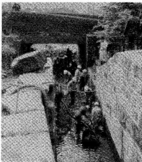
Silted up channel at tail of Lock 31W under Ward Lane. photo: Bob Dewey
