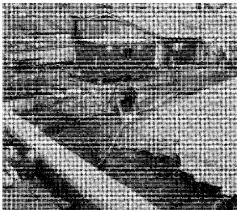
Showing work in progress at Whitelands Rd. looking towards the Ashton Canal.
