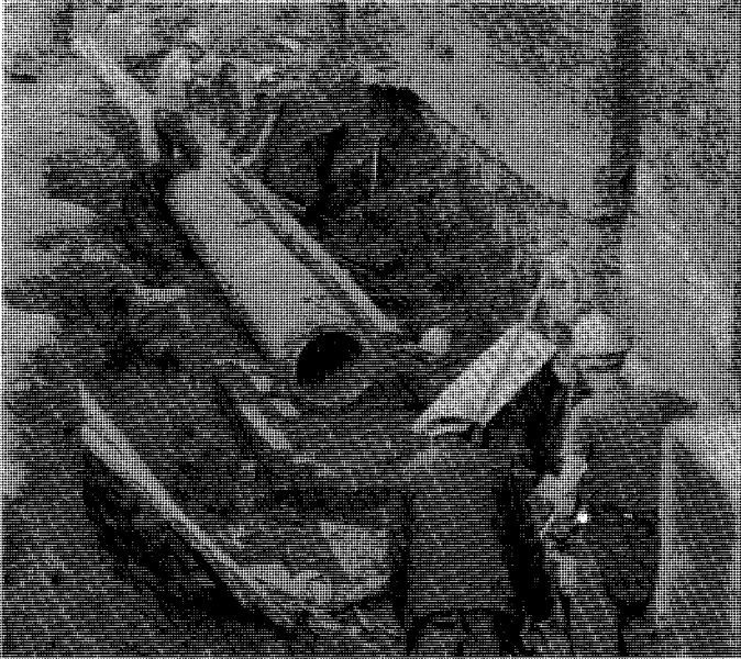
Photo 1: The Society's MSC Community Programme Project — Tameside Canals — is making good progress restoring the canal between Ashton and Stalybridge. Here the concrete bywash pipe is being installed under the towpath at Lock 1 west (Ashton Lock). Shuttering is put in place ready for concreting over the pipe.
