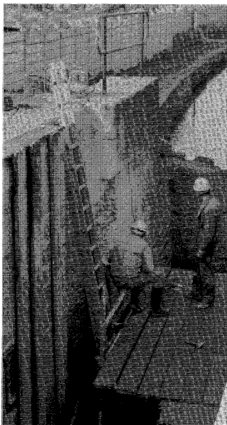
Photo 6: Damaged quoin stones are drilled out at Lock 3 West ready to be replaced. The lock is now complete waiting for lockgates ordered from the Kirklees lockgate workshop.
