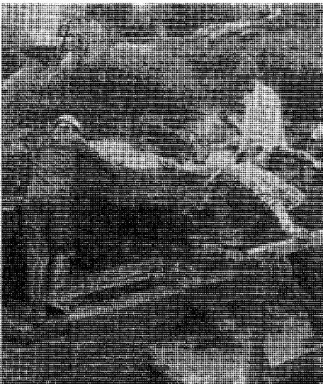
Photo shows rebuilding of tail wall of Lock 31W. Photo: Bob Dewey
