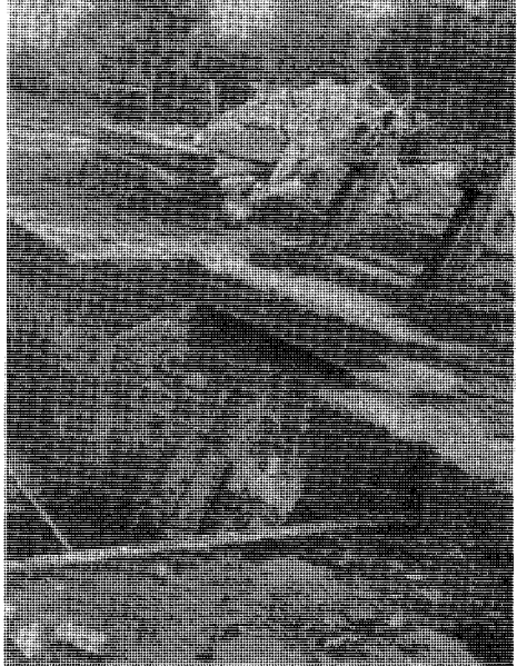
Top of Lock 31W showing sloping paddle gear which had to be concreted in. Photo: Bob Dewey
