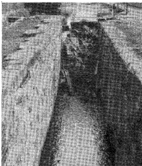
Lock 2 West before work began. Steel pile cap removed and workboat moored at the head of the lock. Photo: Waterways World
