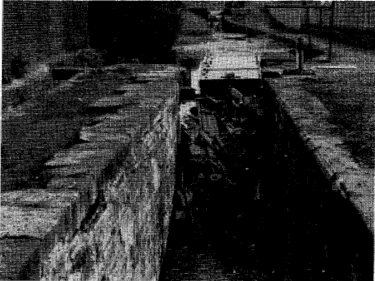
Rubbish collected in the chamber of Lock 2 West. The steel pile cap has been removed, and a work boat is moored at the head of the lock.
