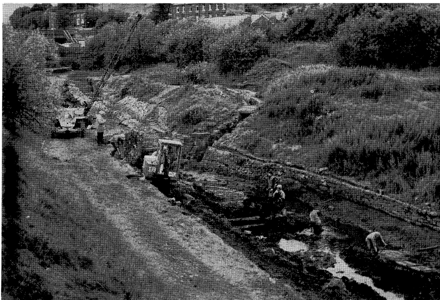
Lock 41E after the removal of the concrete cascade but still before the removal of the infill material from the lock chamber. The bywash is cleared and work has begun in the pound below. The excavator is finishing building a temporary dumper access into the bed of the canal prior to dredging duties.
