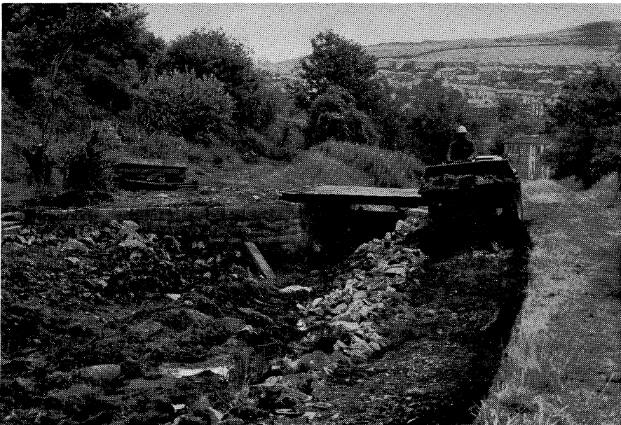
Lock 40E with a temporary bridge over the forebay, and a dumper reversing up the temporary access from the canal bed.
