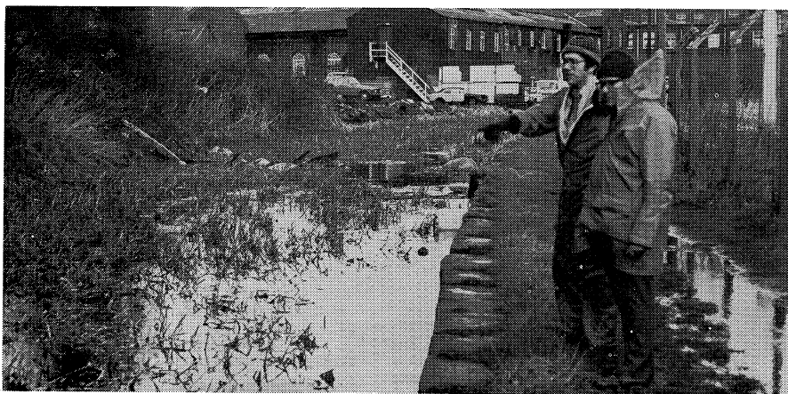
Photo by David L. Finnis shows County Cllr. John Sully and Society Chairman David Sumner (left) looking at a derelict stretch of canal below Bailey Street, Stalybridge.
